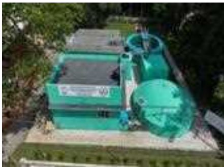
360 KLD STP at General Hospital, Thrissur
