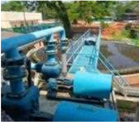
500 KLD STP at Kozhikode medical College
